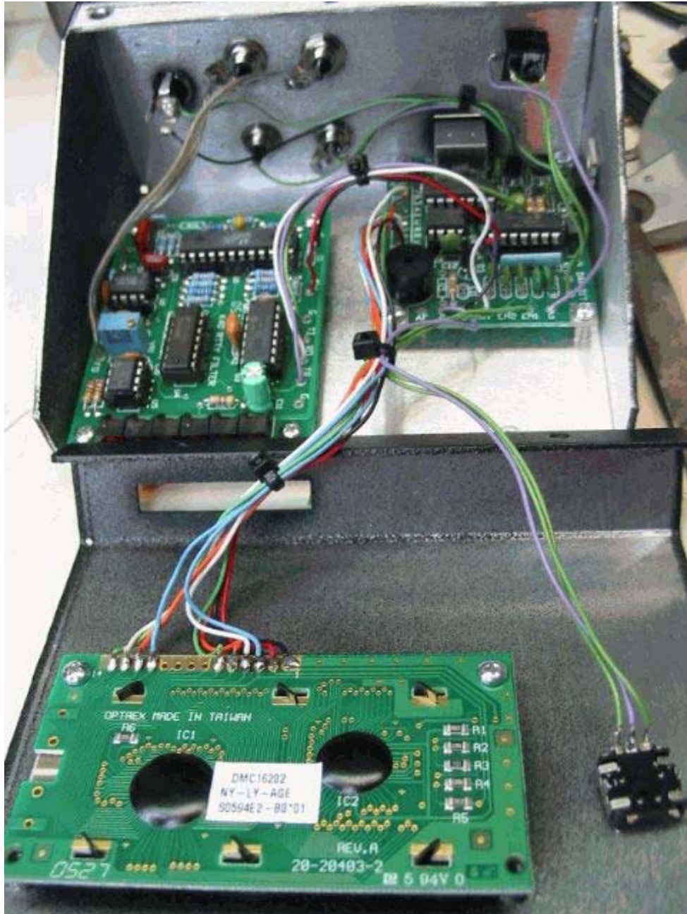
Fig 10 – Wiring Harness to LCD and Speed Control
